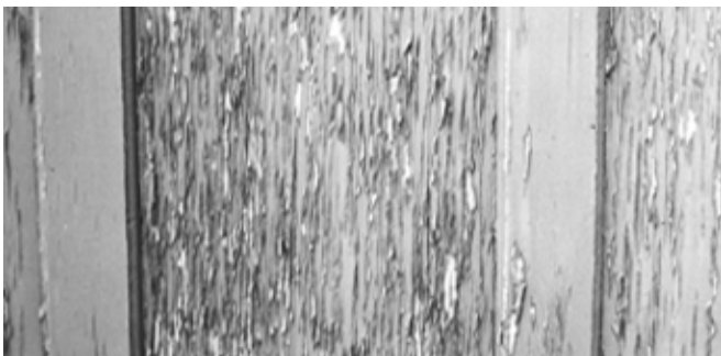
Figure 15-4. Early paint failure on plywood caused by penetration of moisture into surface face-checks.
