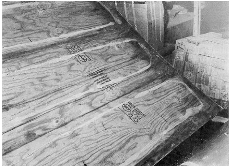
Figure 5.—Plywood back of a collector panel badly water stained due to condensation.
