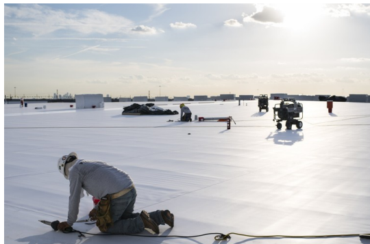
Workers on the job in Garland, Texas, for the King of Texas Roofing Co. last month. PHOTO: MATTHEW BUSCH FOR THE WALL STREET JOURNAL
