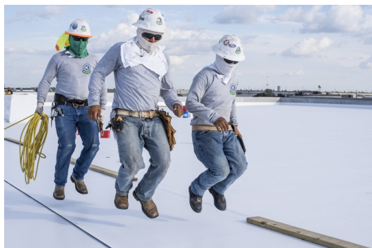
Workers flatten a section of roofing by simultaneously jumping on it. PHOTO: MATTHEW BUSCH FOR THE WALL STREET JOURNAL
